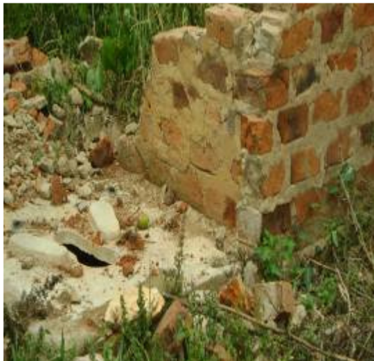
A pit latrine that collapsed in Kakunyumunyu primary school and the Pallisa District authority effected all Payment to the contractor
