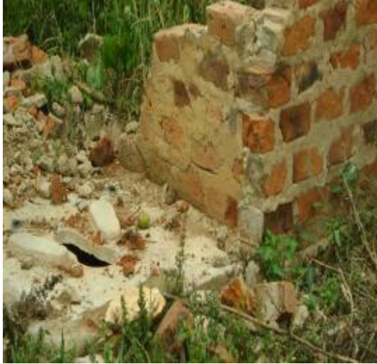
A pit latrine that collapsed in Kakunyumunyu primary school and the Pallisa District authority effected all Payment to the contractor
